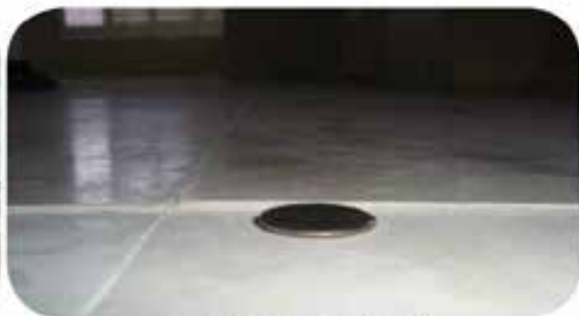
LIPPAGE (UNEVEN TILES)
