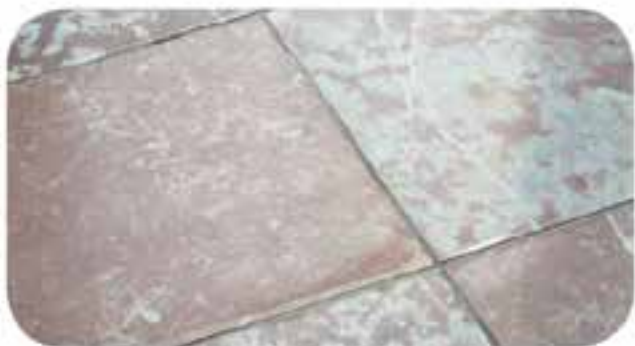
DIRTY, STAINED GROUT LINES
